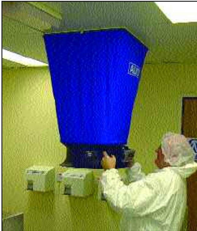
Figure 1 Measuring hood being used to measure the air supply volume in a cleanroom
